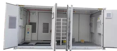
1075KW HH ESS
