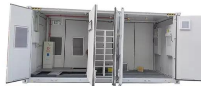
1075KW HH ESS
