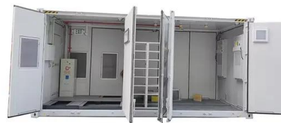
1075KW HH ESS
