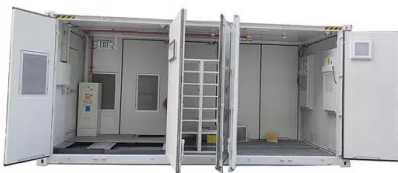
1075KW HH ESS
