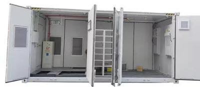
1075KW HH ESS
