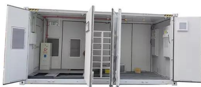
1075KW HH ESS
